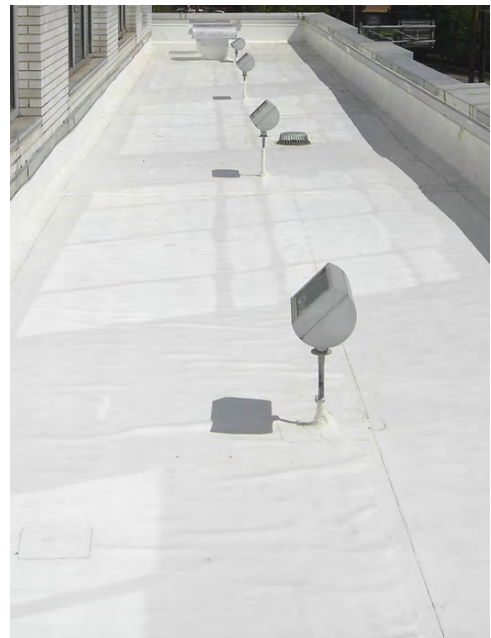
White single ply roof, cleaned and ready to be coated with AlphaGuard.
