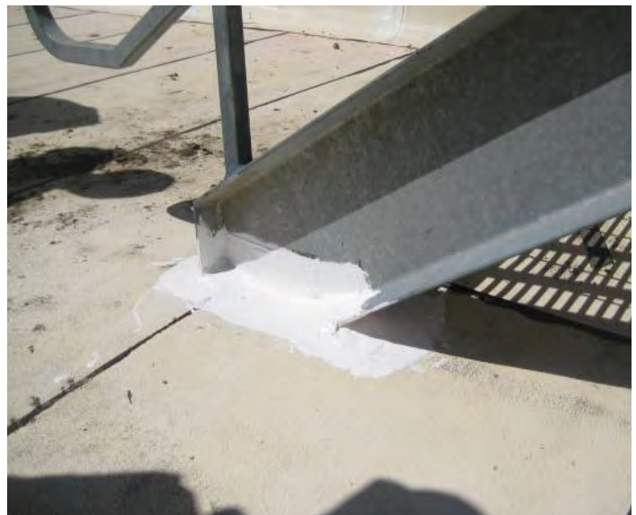
Penetrations that previously needed pitch pockets are flashed with AlphaGuard. This eliminates possible points of water infiltration.
